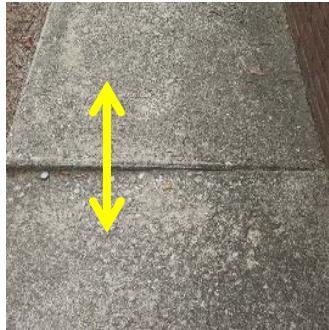
1/4 to 1/2 inch change in sidewalk level
