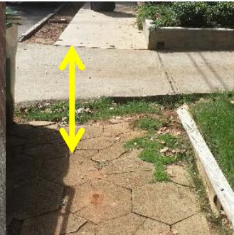
Over 1/2 inch change in sidewalk level
