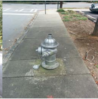
Example of horizontal sidewalk obstruction
