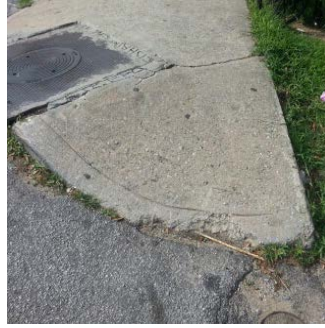
Ramp Present, doesn't meet ADA Standards
